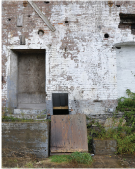
Building scars on west facade.
