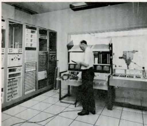
Figure 2 - The television control room demonstrating the equipment racks which are being installed, and the video and audio switching consoles. A small studio and camera is visible through the sound-proof window in the background.
